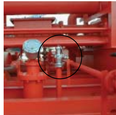
View of Installation Shut On/Off Valve Model : TVC-02
